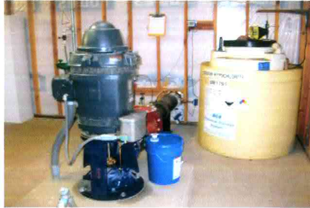
New well At Family Park -- complete with electronic controls and automatic generator back-up.
